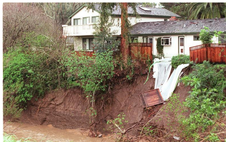
Photo 1: A house on Bay Laurel Drive in Menlo Park lost its fence to the eroding bank of the San Francisquito Creek on Feb. 19, 1998
