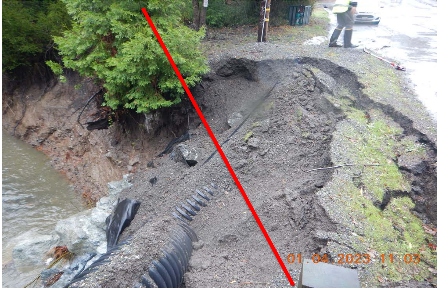
Embankment Erosion Northeast
