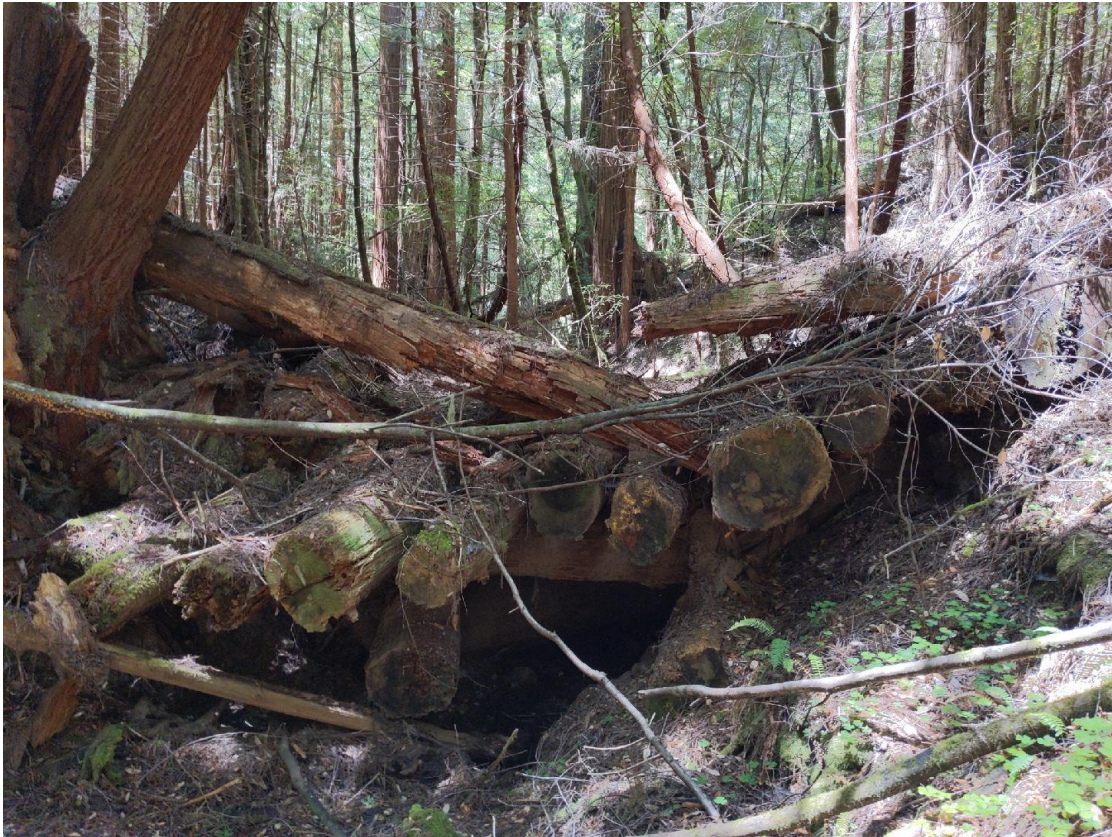
Figure 12 A failed, historic "Humboldt crossing" on an ephemeral stream, PCCP
