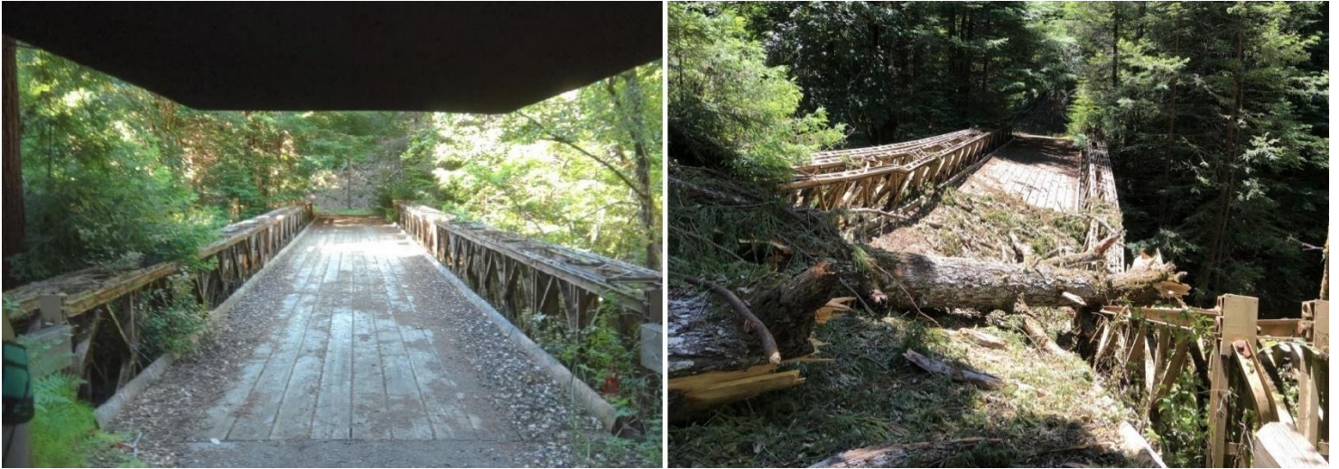
Figure 7 Baker Fire Road Bridge before (left) and after (right) tree damage
