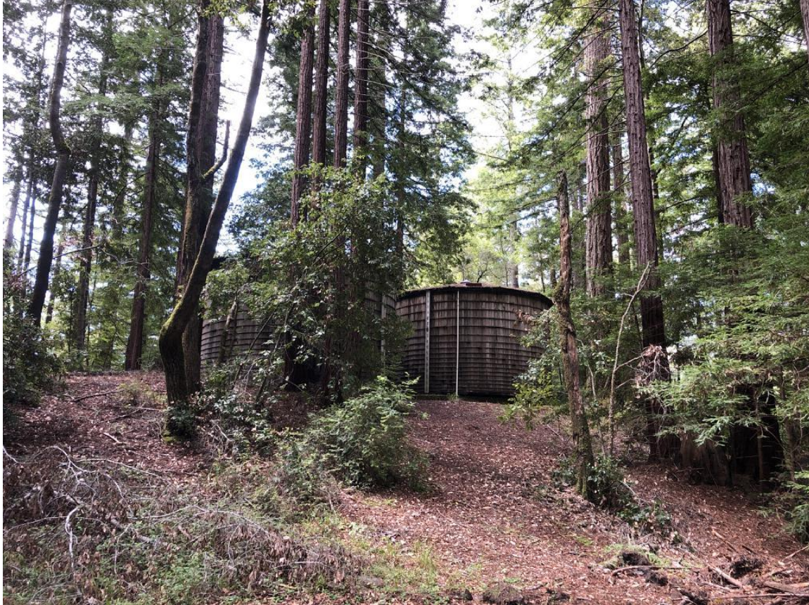
Figure 10 Existing water tanks above Honor Camp
