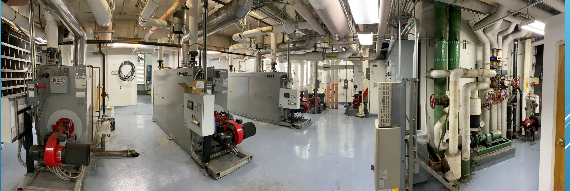
HALL OF JUSTICE AIR HANDLING UNITS
