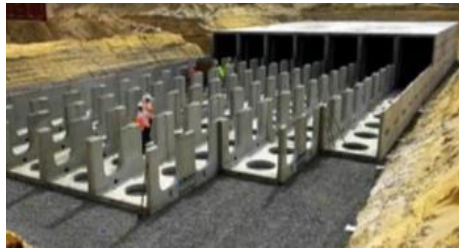
Figure 1.12. Subsurface infiltration system (under construction), Sun Valley Park, Los Angeles. (Source: Conteches.com)
