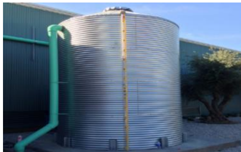
Figure 1.14. Rainwater harvesting cistern, Environmental Innovation Center, San José. (Source: City of San Jose)
