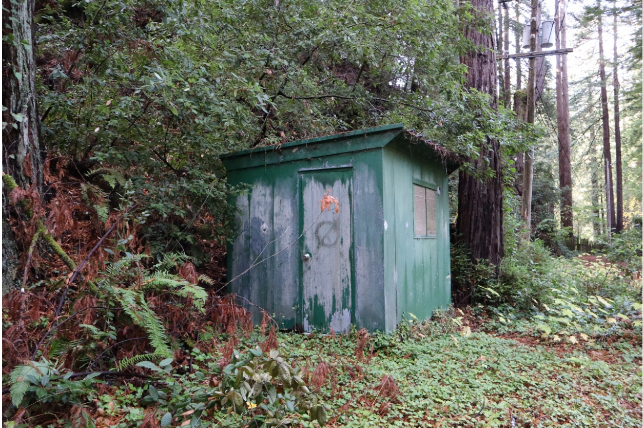
Photo 19: Cabin Site – Pump House
